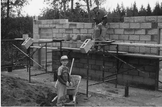
Door jambs were put in place for the restroom building by Tom Permenter, Joe Putnam, and Ken Bloom.
