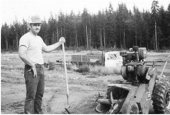
Bill Bergthold with his equipment installing the sprinkler system for the athletic field located near the south boundary of the park.
