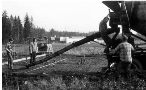
Mark Myres, Ken Bloom, and Keith Iverson pouring the restroom building slab.
