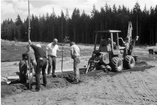
Curt Gordon, Hanford Thayer, Jim Porter, Ryan Porter, Pete Krogseng, and Bill Bergthold placing drain pipe in trenches.
