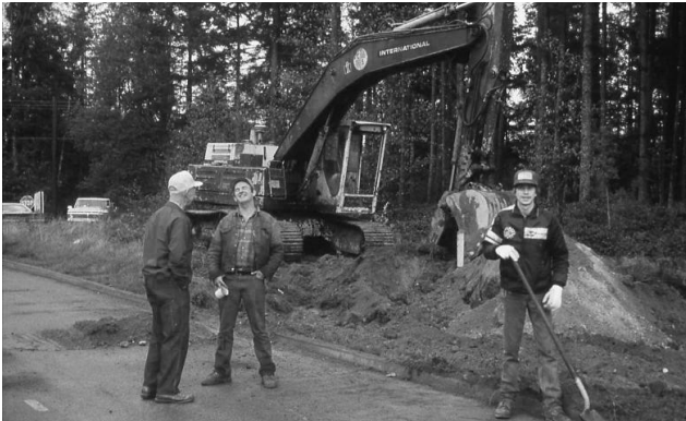
Excavating the remaining portion of the easement donated by Arthur (Johnny) and Dora Gabelein.
