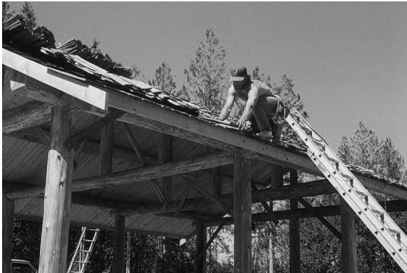
Dave Johnson is shown putting shakes on the roof of the picnic shelter.
