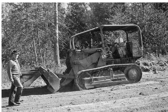
Jim Scriven donated his bulldozer to excavate the site for the restroom building. Hanford Thayer is on the left.
